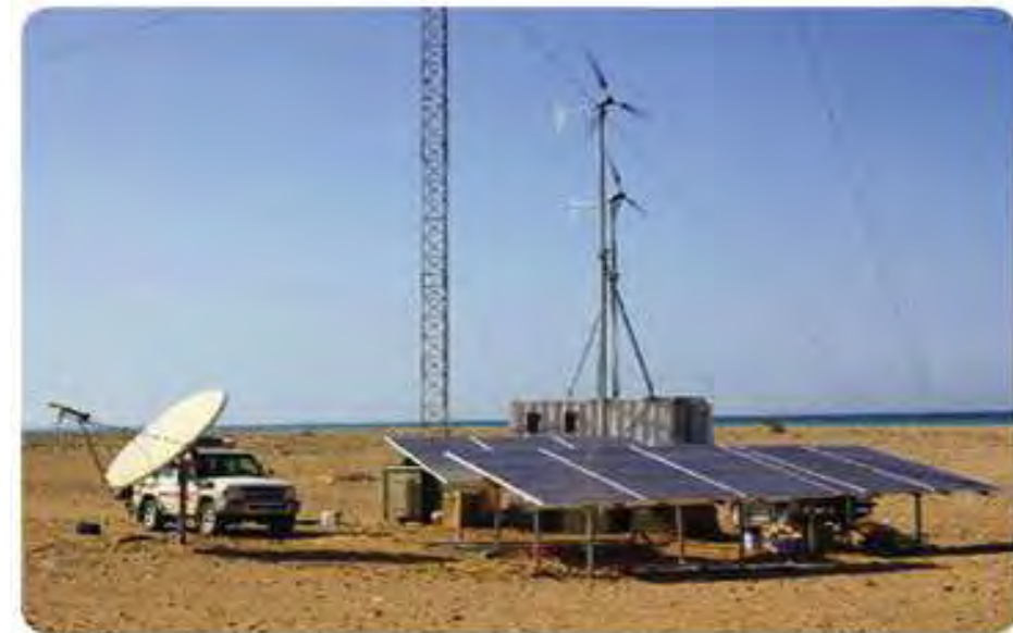
e.g. power supply for mobile phone stations
